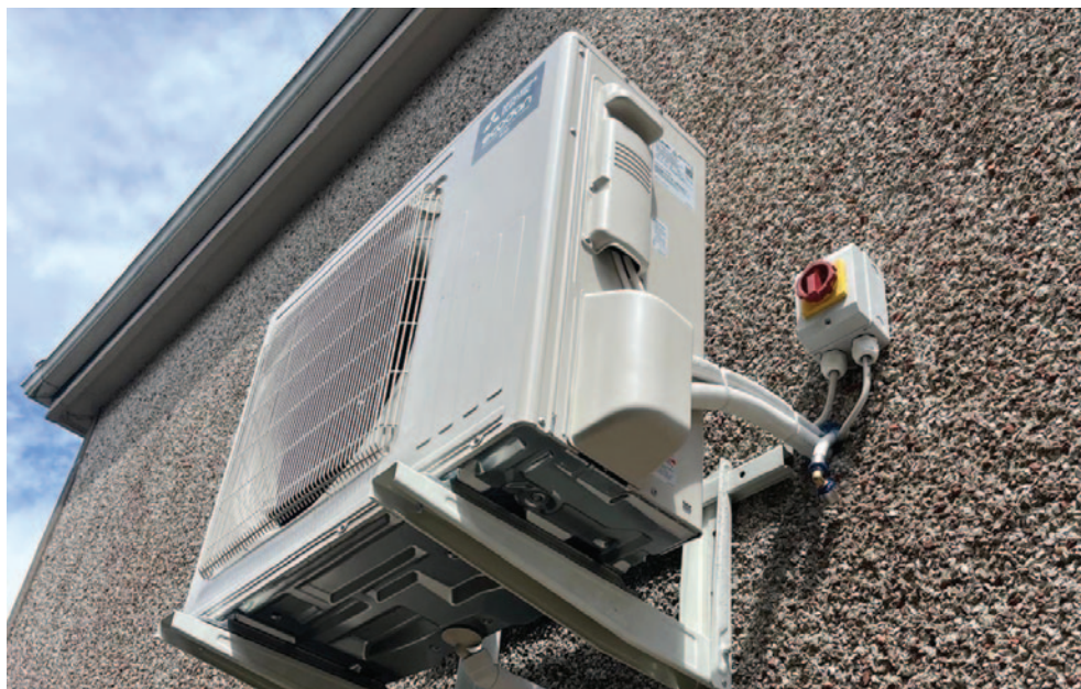
An air-to-water heat pump installed at a home as part of an energy upgrade.
