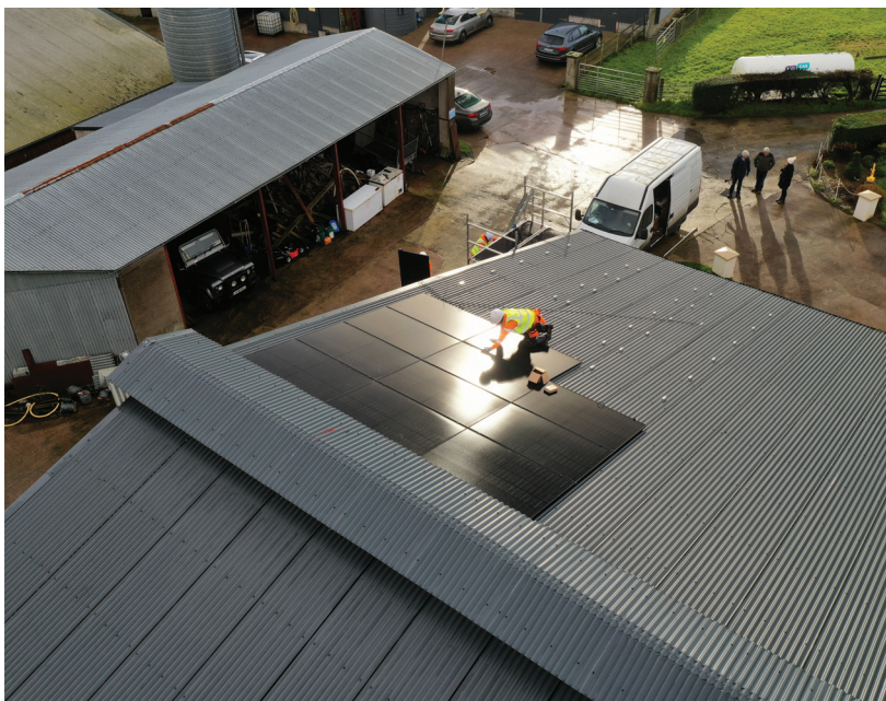
Bord Gáis Energy's innovative partnership with the IFA is bringing solar rooftop installations to farmers across Ireland.
